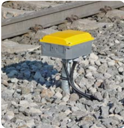
Metering device cabinet
