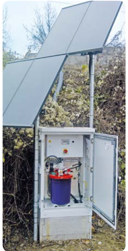
Solar unit with battery storage
