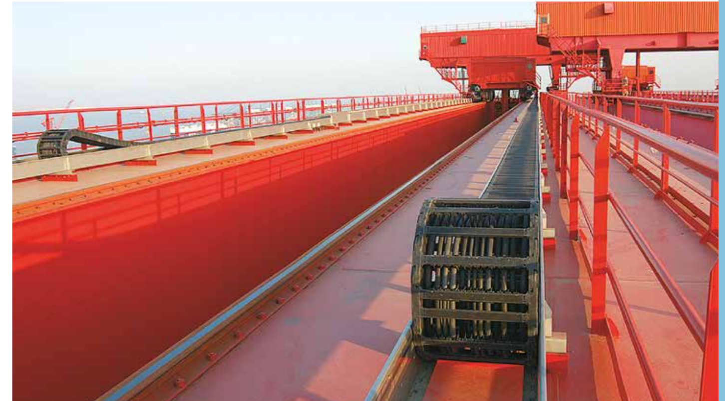
Shipyard crane: travel 180m, weight 30kg/m: since installation in 2001, this igus® E4/4 rol e-chain® has run trouble-free in spite of severe weather conditions. Even a typhoon did not cause any operating problems
