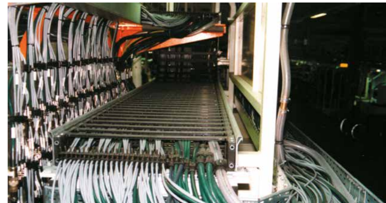
chainflex® CF5 and CF6 control cables (green) as well as CF211 measuring system cables (grey) in a screwing station of a car factory. e-chain®: E4/00 system with chainfix clip strain relief devices.
