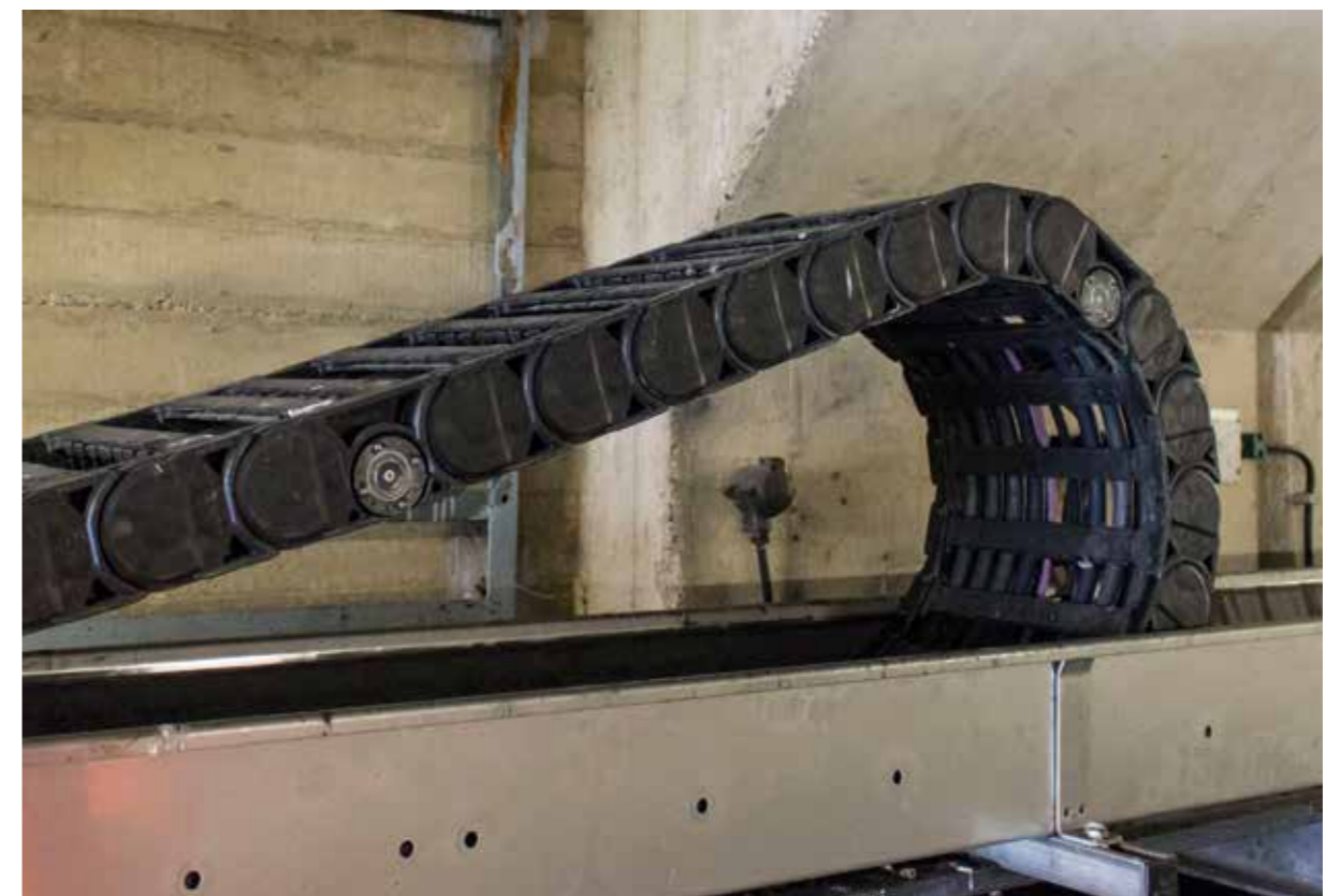
chainflex® fibre optic cable in a sea lock
