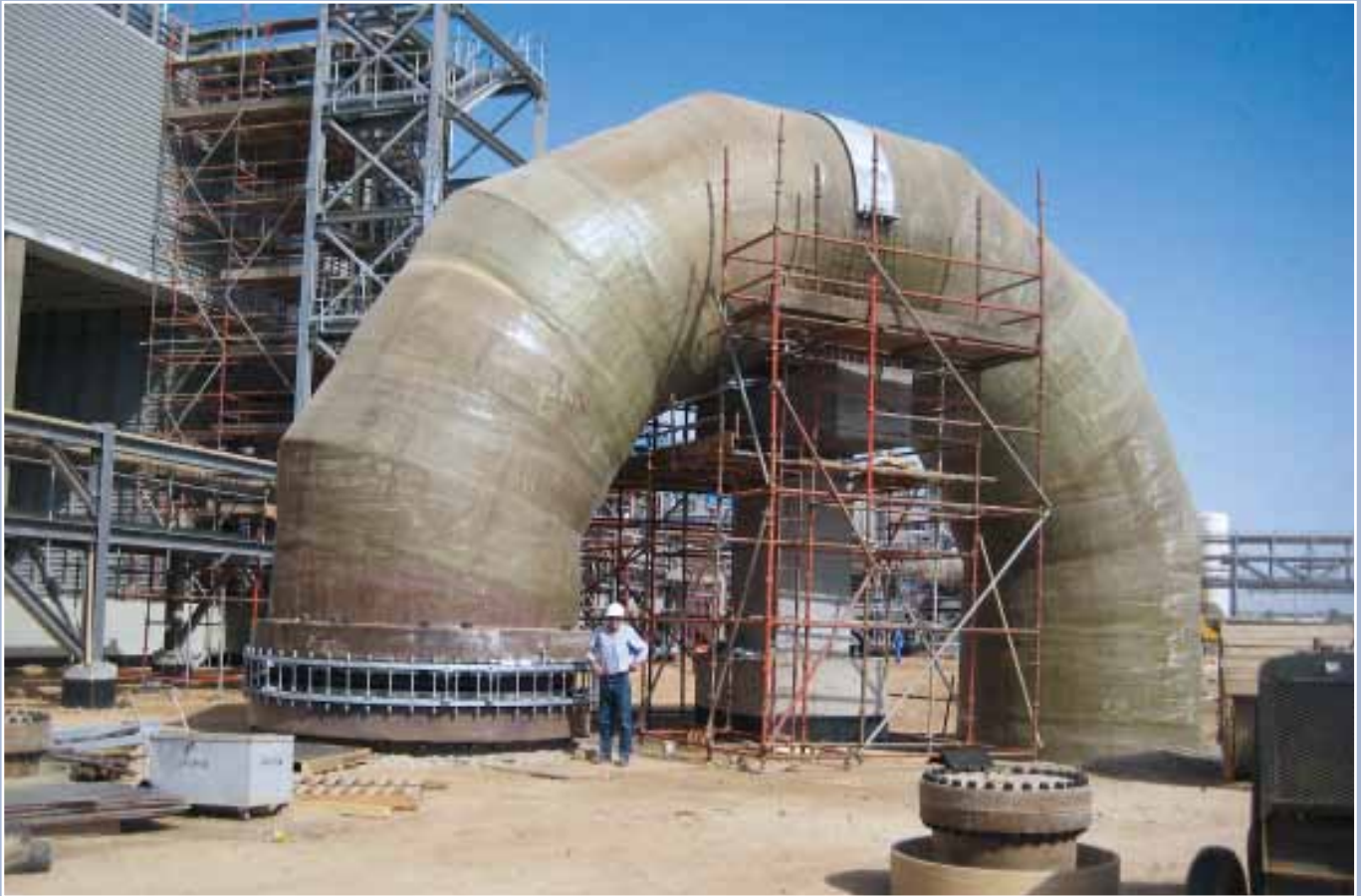
Type U110M lateral expansion joint in a desalination plant NB 3600, 8 bar, 90°C
