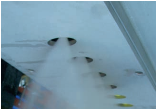
Sprays in operation with cover plate on
