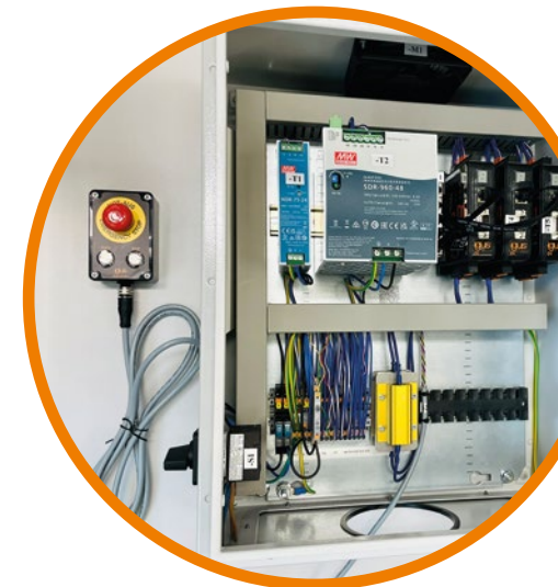
Switch cabinet installation with freely positionable external emergency stop switch
